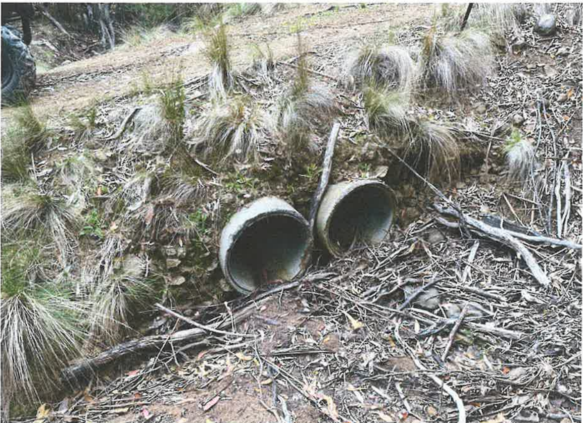
Photo 10: Field photo showing existing culvert on the proposed property access to Lot 1.
