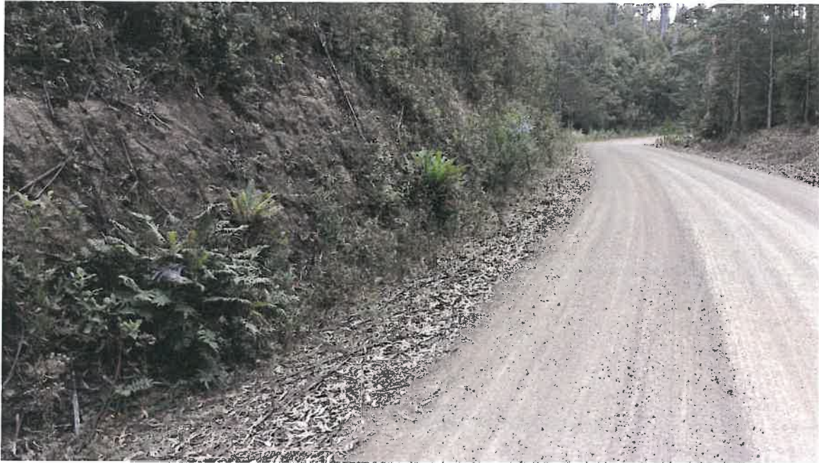
Figure 2 – Road surface rated as requiring reduced overlay thickness of 75mm
