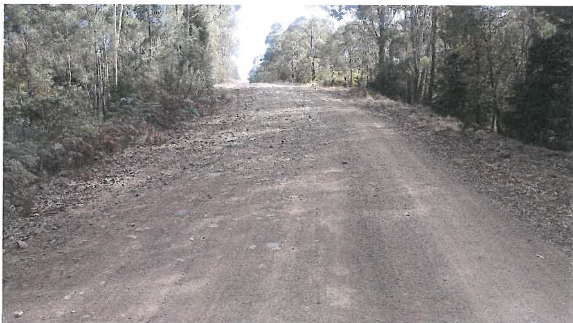
Figure 3 – Road surface rated as requiring 100mm overlay
