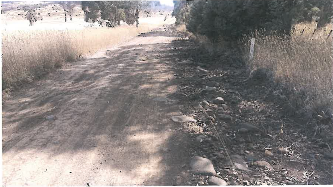
Figure 4 – Road surface rated as requiring 150mm overlay
